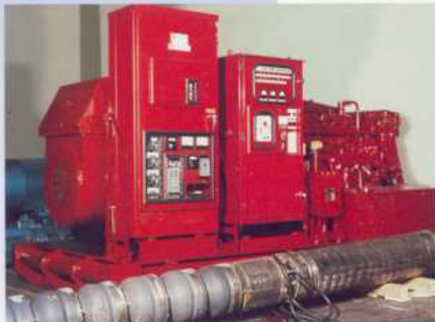
Electro-submersible fire pump with dedicated diesel gen-set.
